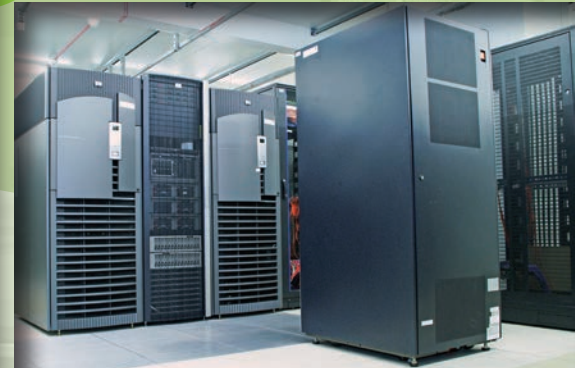
ZUS servers support one of Europe's largest information systems. ZUS collections
